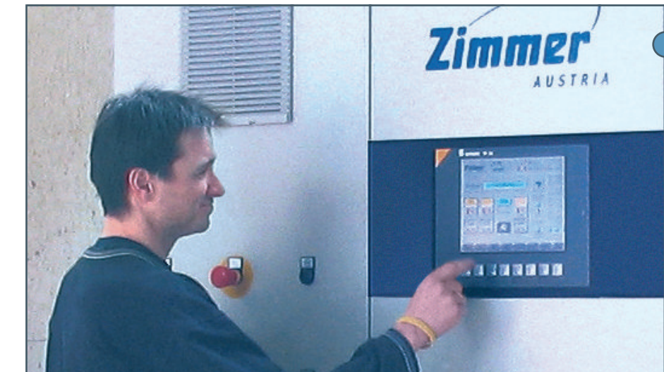
Central automation PLC-unit
